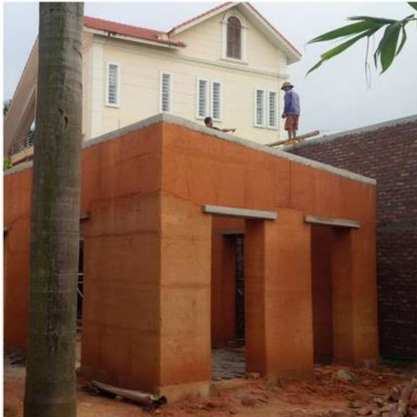
6. Completed wall with overhead elastic interstices; wall capping to be locked by concrete brace (thickness 150) along the wall
