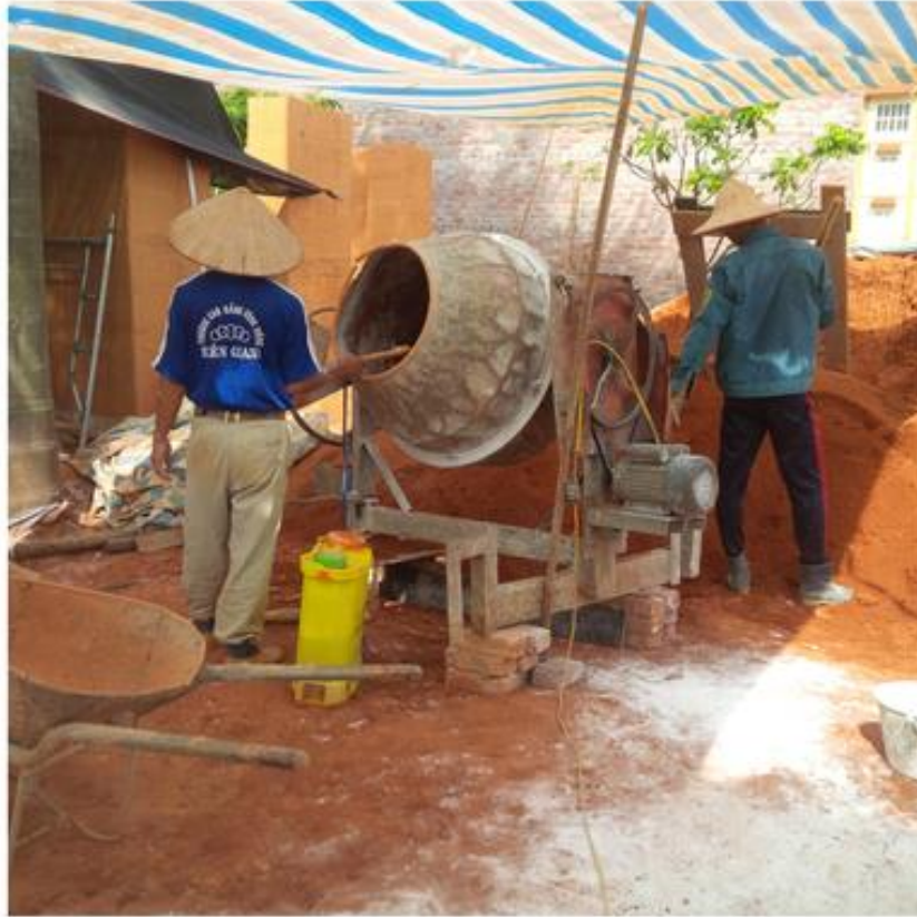
1. Locally available earth to be ground and mixed with additives to improve the earth hardness
